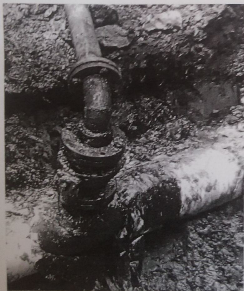
Fig C: SPILL POINT WITH 4" VALVE INSTALLED
